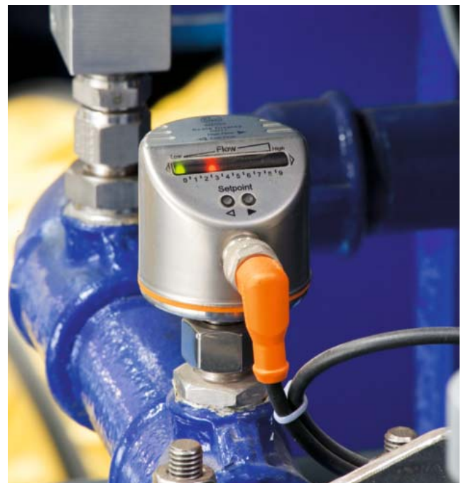
Flow sensor in a cooling water monitoring application.
