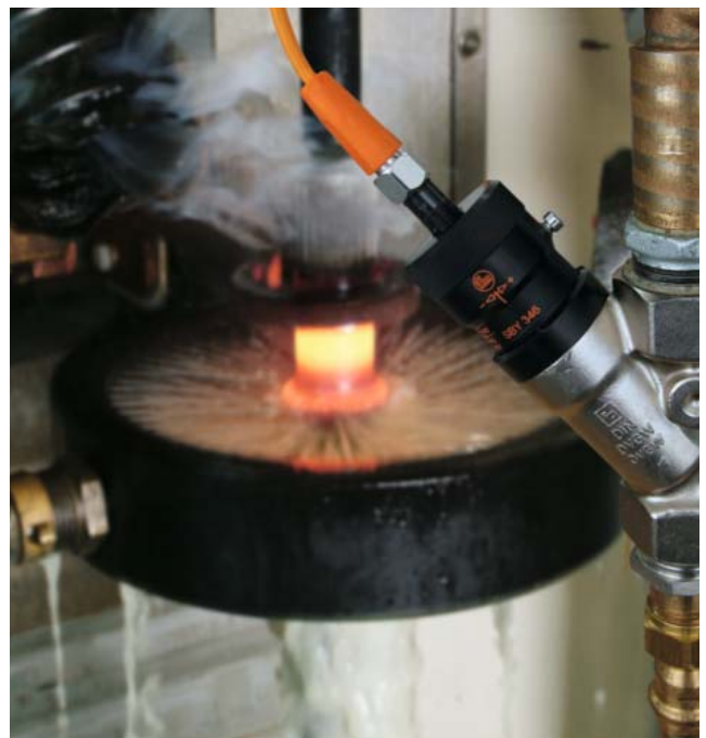
Mechatronic sensor in the coolant circuit of an induction furnace.
