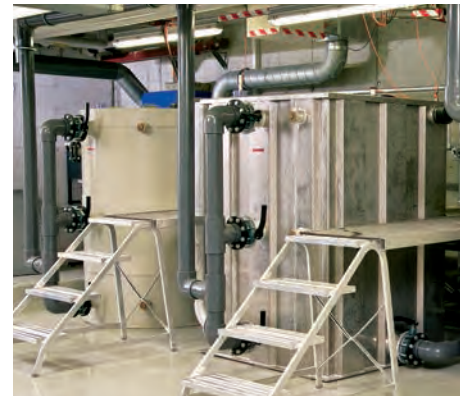
Level measurement in a water treatment plant
