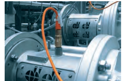
Accelerometers type VSA are connected to VSE units to monitor critical components of the process (pumps, motors, agitators).
