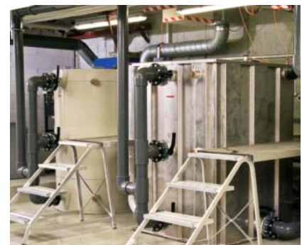
Level measurement in a water treatment plant
