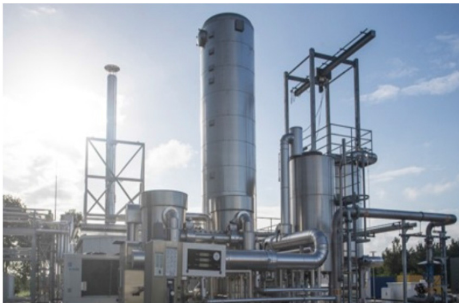
Fig. 2 Power-to-Gas Plant to Produce E-Gas
