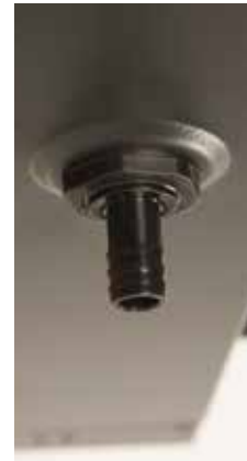
Condensation-water discharge fittings
