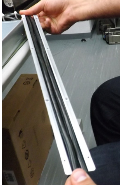
Figure 33: Cables within the Rail
