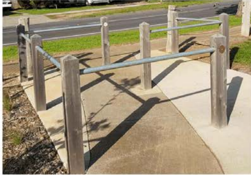
Chicane style pedestrian access – generally installed reserve path access points
