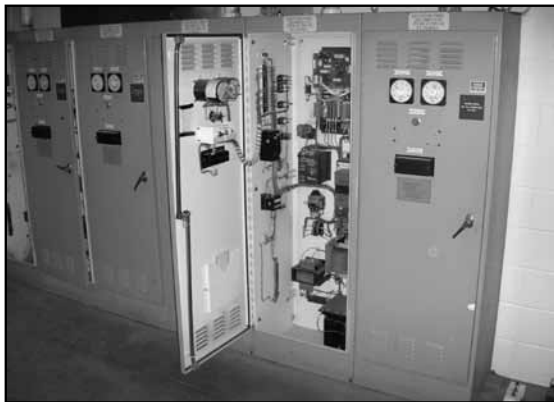
A typical '80s analog exciter control panel crowded with obsolete components
