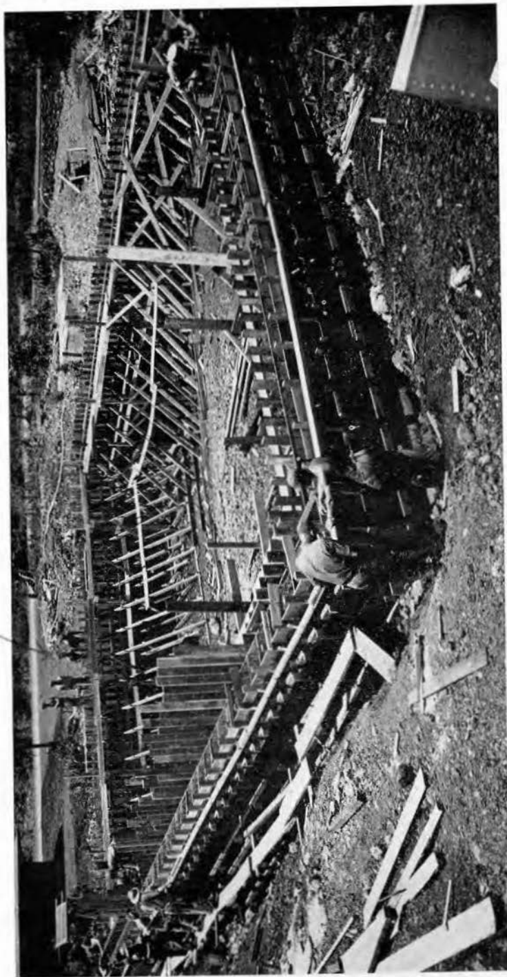
BUSINESS BEFORE PLEASURE The newly completed station swimming pool as it appeared during the early days of its construction.
