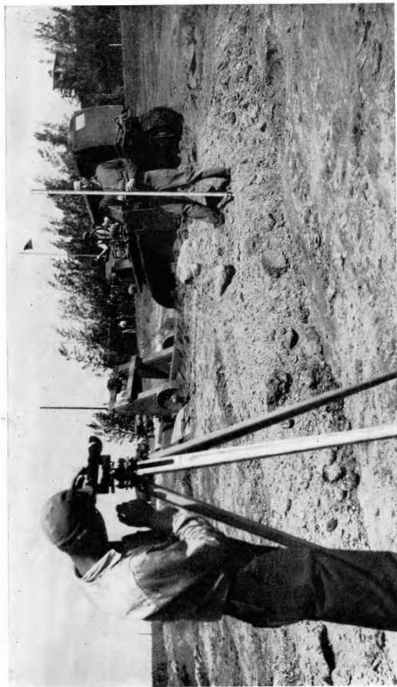
STRICTLY ON THE LEVEL! Members of a surveying party work hand in hand with heavy equipment operators, checking to see that the correct grades are maintained.
