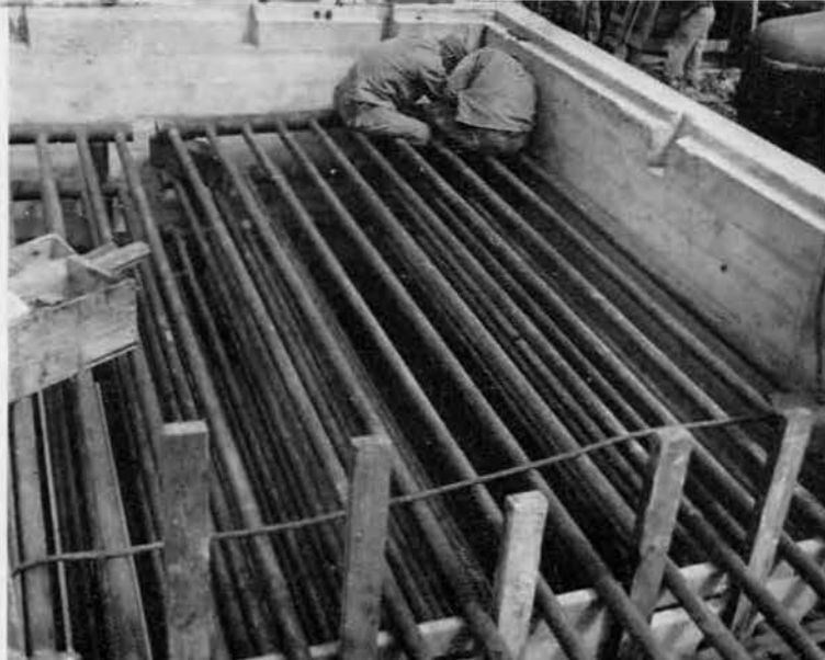
PIPING IN MELTING TANK
