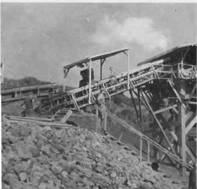
MAIN CONVEYOR AND SPLITTER BIN
