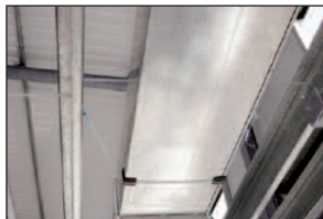
Square Air Ducts
