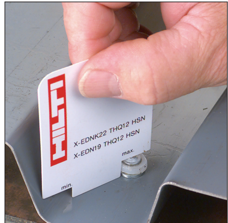
Checking the standoff of an X-EDN 19 roof deck fastening with a plastic template
