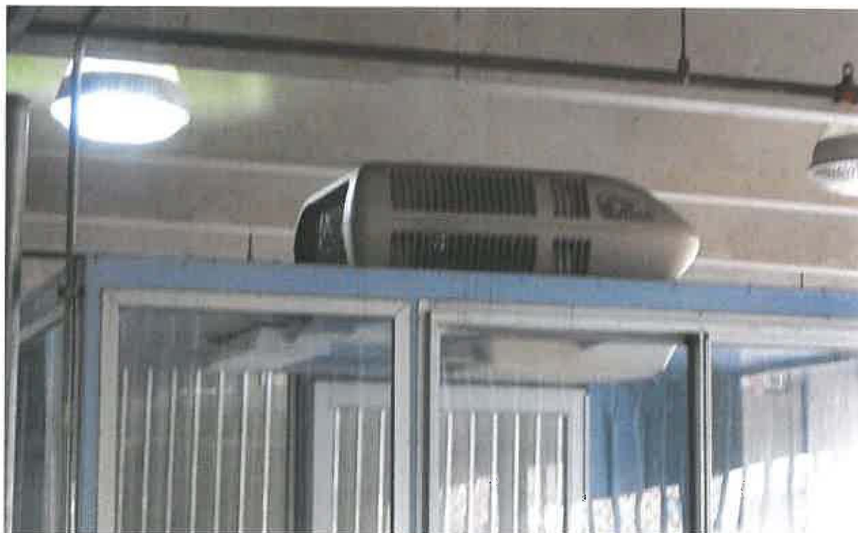
Parking Garage, Guard/Parking Attendant Station, Coleman Mach
