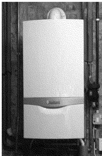
Figure 7. European gas boiler
