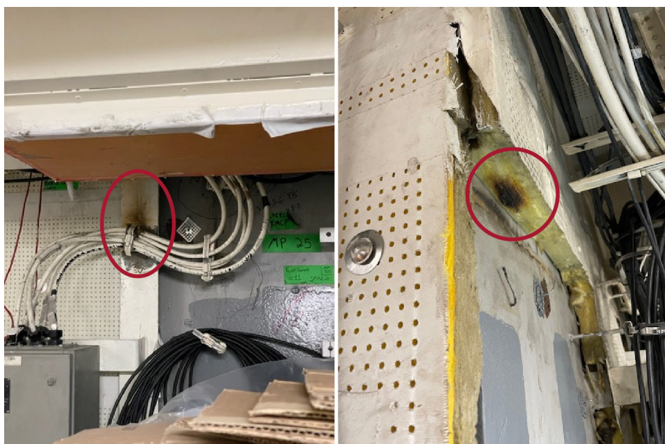
Figure 5: Damage from Two Unreported Hot-Work Incidents
