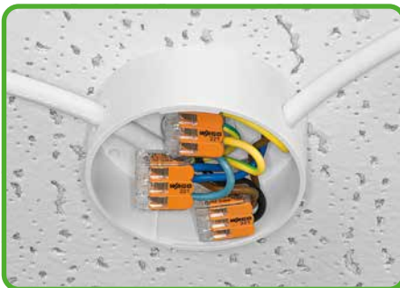
Lighting distribution in ceiling canopy
