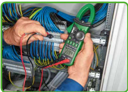
Voltage testing in switchgear cabinet
