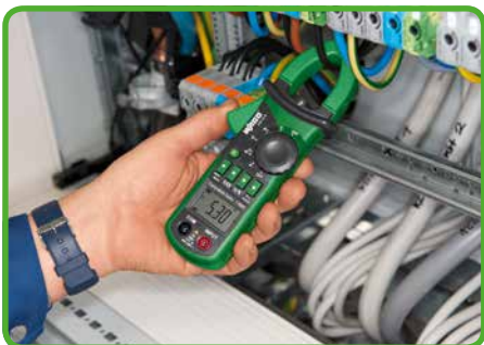
Current measurement in switchgear cabinet
