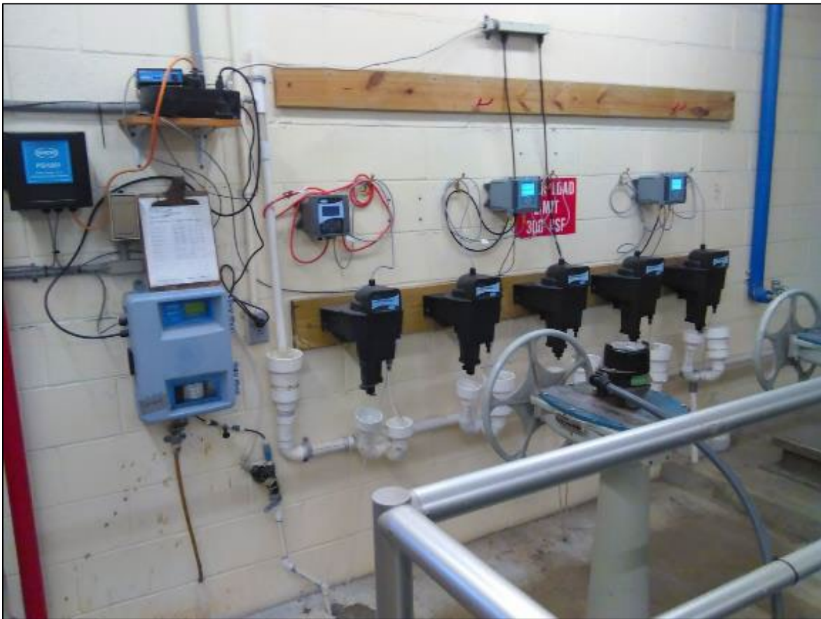
FIGURE 22. Online turbidimeters with SC200 controllers on the operating floor of the filter gallery.
