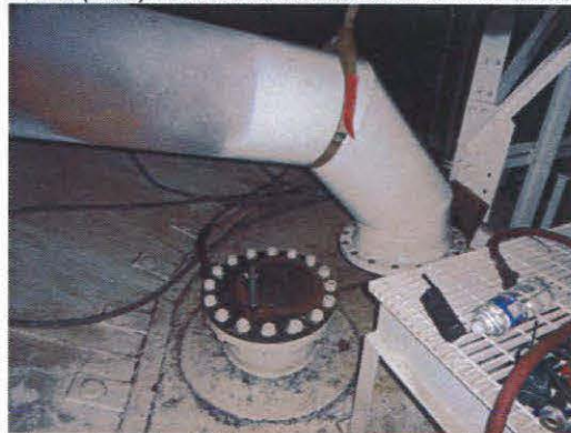
Figure 3.0: The 18" line was prepared for testing by removing the diffuser and installing a ported blind on the pipe flange as indicated. This connection was a standard ANSI Class 150 flange.
