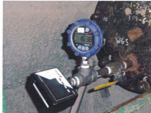
Figure 5.0: As a precaution against possible air entrapment, we removed our test tree and connected the test instruments directly to the pipe in an effort to stabilize the pipe. The efforts were not successful.
