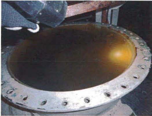
Figure 10.0: The 32"Ø pipe was drained just enough to remove the flange to change the gasket. We confirmed that there was little room for trapped air at this point.
