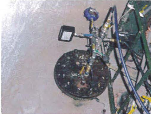
Figure 4.0: Test tree on the 12"Ø flange in the lower access tunnel for the 18"Ø line.
