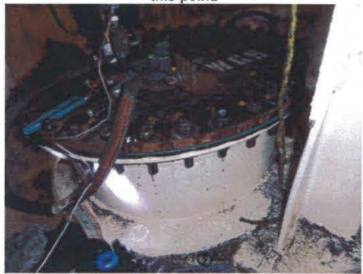
Figure 12.0: One of the failed attempts at pressurizing the 32"Ø line. Note active leaks form the bolts due to the gasket not ssealing.
