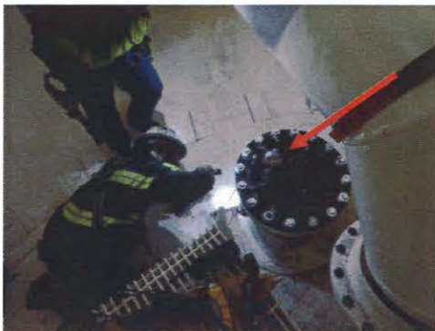
Figure 6.0: The 18"Ø line inside of Tank 5. Note temperature probe connected to the port on the blind flange.
