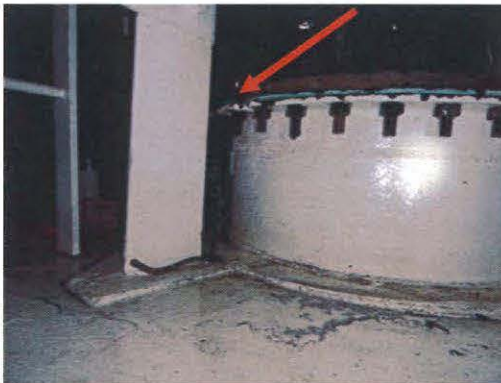
Figure 8.0: There was a small notch cut from the flange of the 32"Ø line inside of the tank. This notch was the source of some of the leaks that proved difficult to overcome on the 32"Ø flange.
