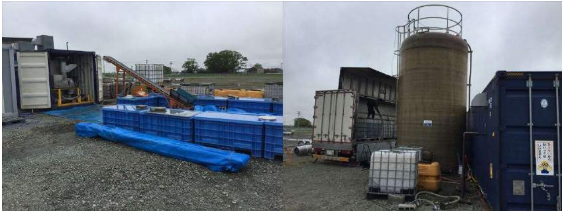
Vegetable waste based biogas digester in Watari cho, Miyagi prefecture
