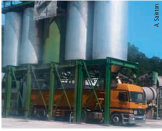
Photo 1 Centrale d'enrobage VALSE Valse asphalt mixing plant
