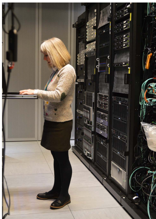
Detail from the Genome Campus data centre, with Dawn Johnson, data centre engineer..
