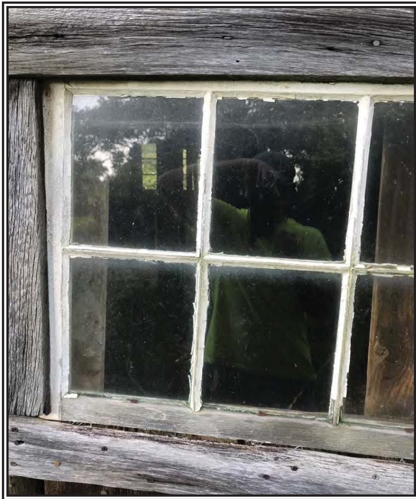
Photo 3: Asbestos-containing Window Glazing Compound
