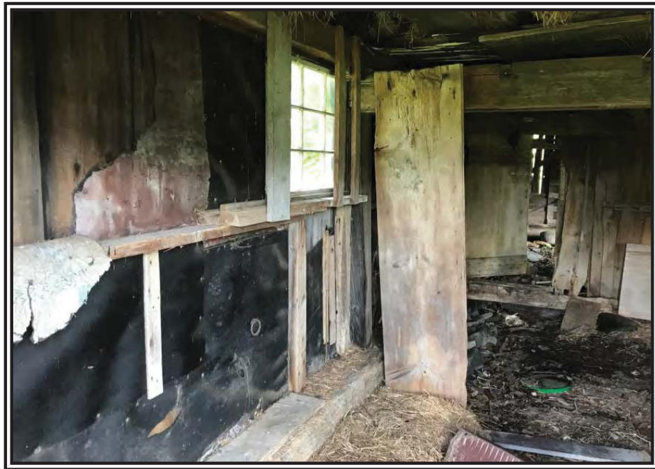
Photo 2: Non-Asbestos Top/Bottom Shingle (Weathered) and Tar Paper under Shingle – Interior Wall
