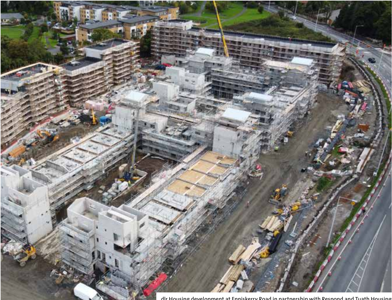
dlr Housing development at Enniskerry Road in partnership with Respond and Tuath Housing
