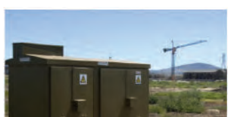
Monitoring of the Electrical Network
