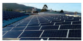
Monitoring of Solar Installations for Self-Supply
