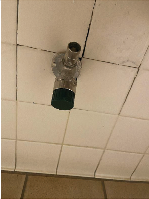
Photo #5: Hose bib located under sink in restrooms
