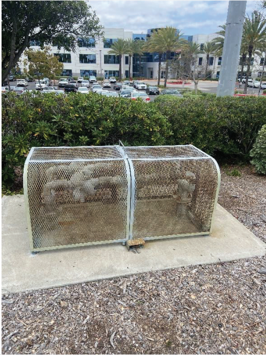
Photo #1: Municipal water connection
