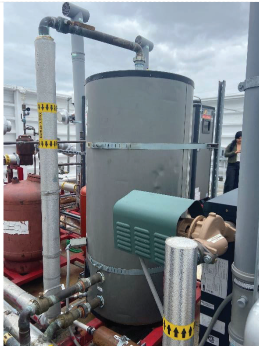
Photo #4: DHW Storage Tank
