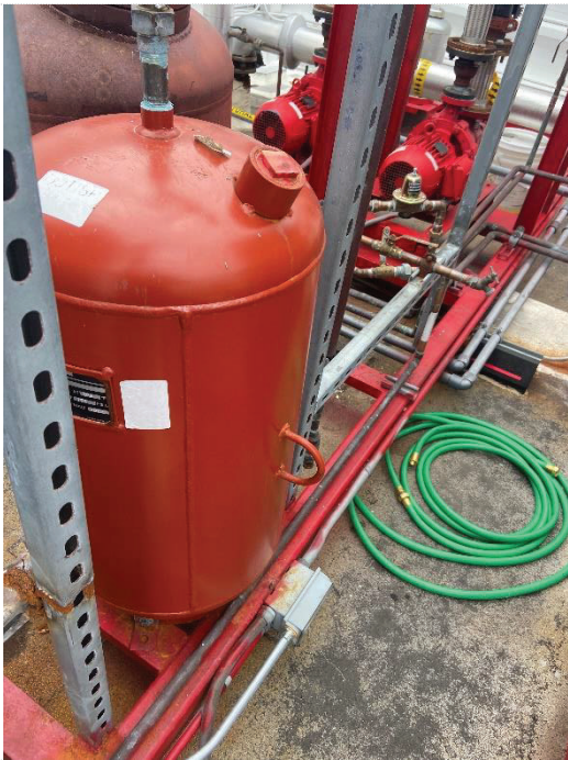
Photo #3: DCW Expansion Tank
