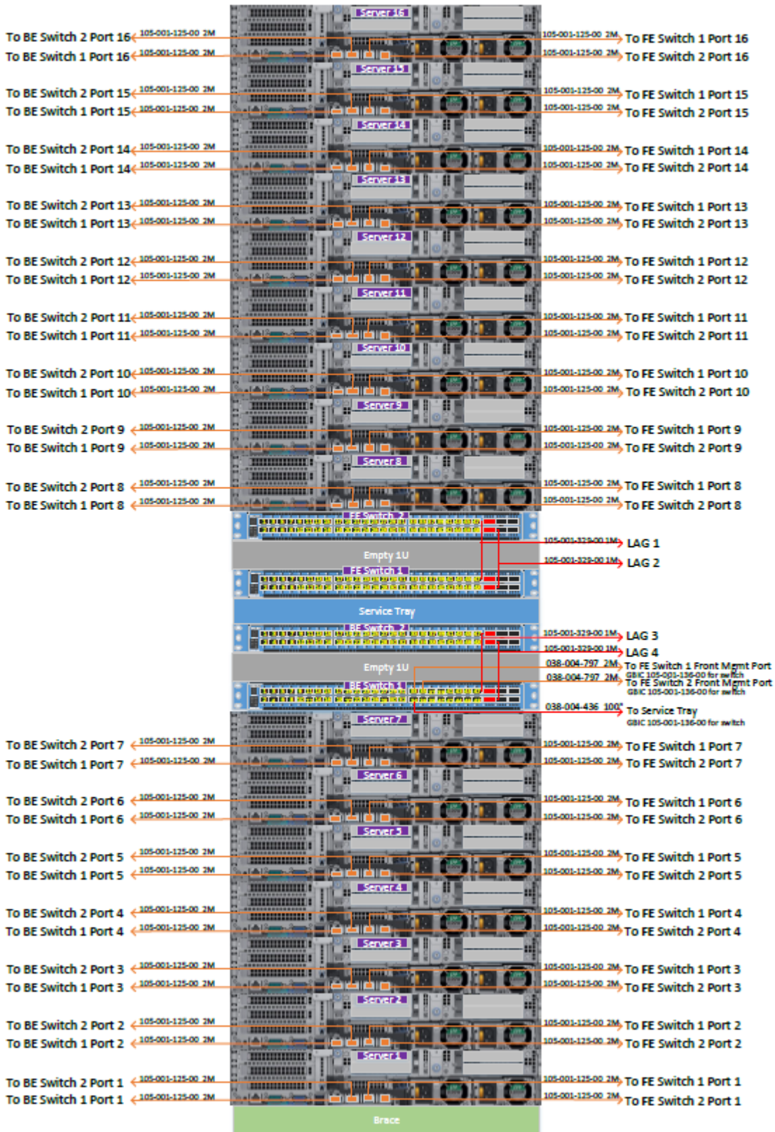
Figure 57 EX300 network cabling
