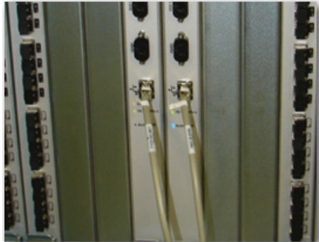
Figure 44 Connecting the ethernet cables (1 director)
