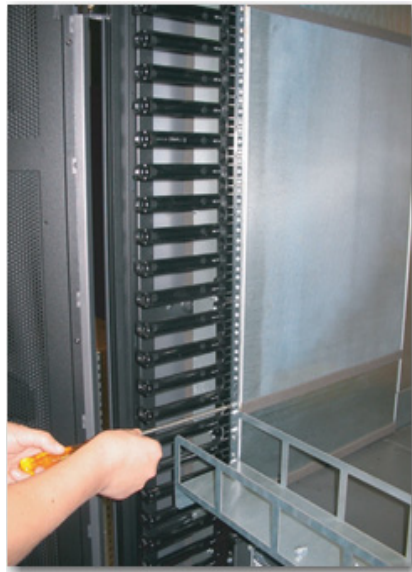
Figure 58 Removing the 14 U baffle
