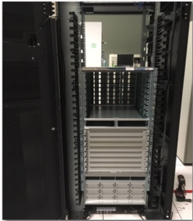
Figure 66 EC-1700 cabinet with MDS 9718 directors installed
