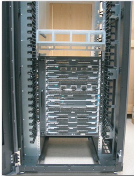
Figure 46 MDS 95XX installed in lower cabinet position
