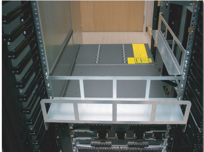
Figure 47 Lower cable tray
