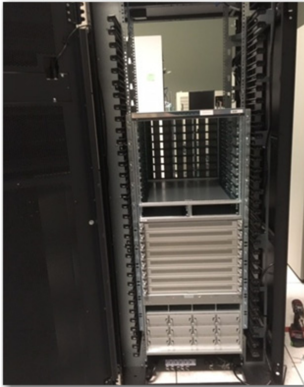
Figure 65 MDS 9700-cabkit installed in cabinet position
