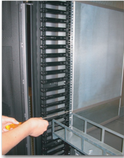
Figure 48 Removing the 14 U baffle
