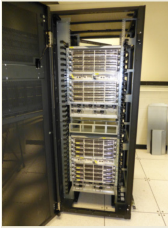
Figure 61 EC-1700 cabinet with two MDS 9710 directors installed
