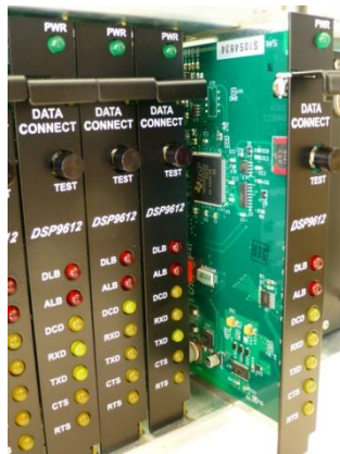
Figure 2-4. Modems Installed in the Rack
