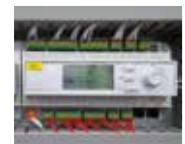
Controller box upgrade
