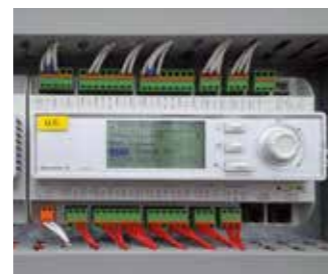
Controller box upgrade
