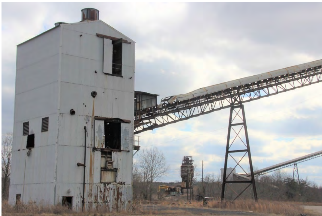
One of the tipples used to feed stockpiled coal to the wash plant
