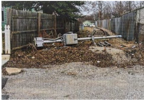
This view of 15 th and Beeler in New Albany, Indiana, shows the condition of the CSXT track on February 19, 2020. (Lee Gordon)
