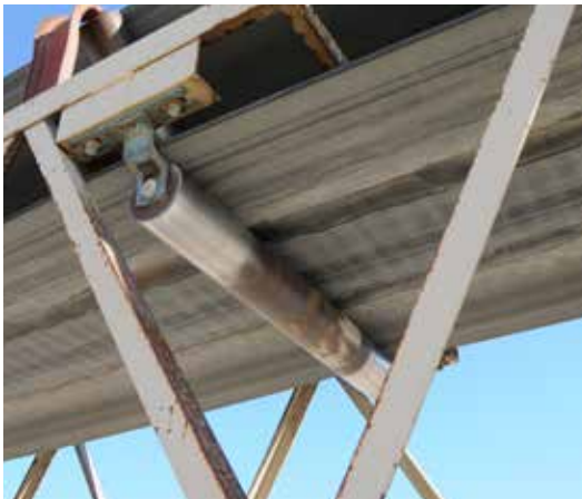
BEFORE: BELT/BACKET DAMAGE
