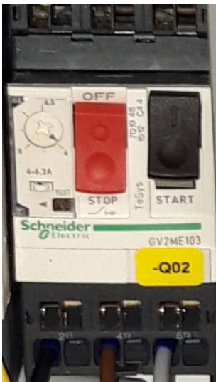
Figure 23: Circuit breaker with overcurrent protection
