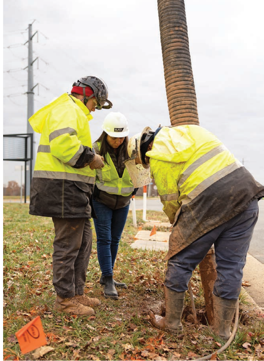
Operator Lawrence Richey digs to locate a utility while operator Annamarie Fagnani and Kristy Black watch the progress.
