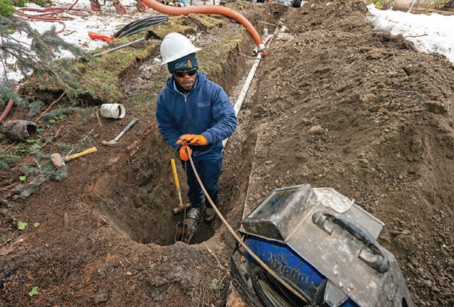
« Jules Matabishi uses a MyTana camera to inspect the old pipe before shooting the liner.
