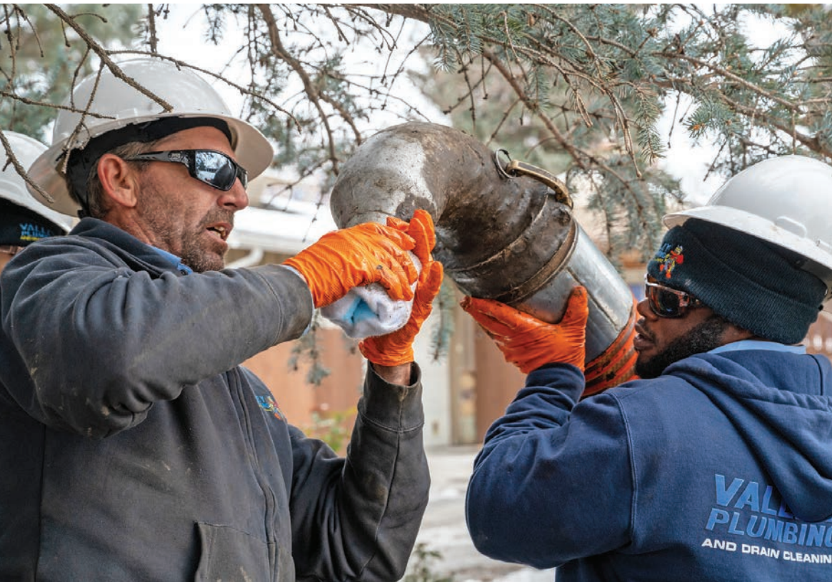
Joey Howard (left) and Jules Matabishi position the end of the liner in the Quik-Shot system before installation.
