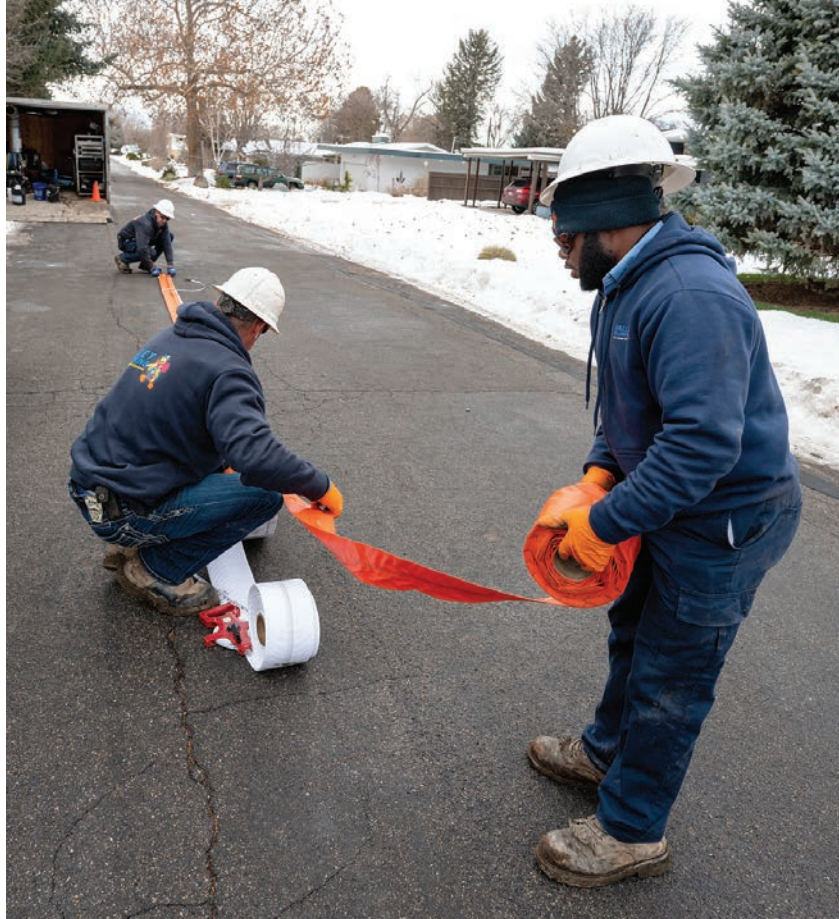
▲ Howard, Matabishi and Sides (clockwise from top) lay out the liner and sleeve and cut them to the correct length.
