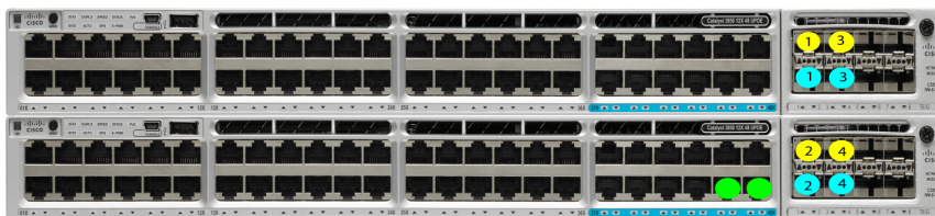
Dual 10/25GE ToR Switches (standalone or stacked)
