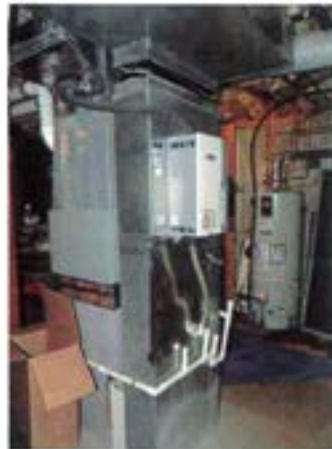
FHA Propane Fired Heat / AC System Basement
