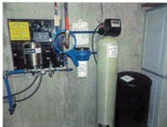
Water Filtration / Well Pump Basement
