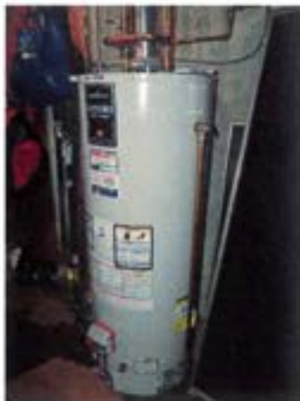
Hot Water Maker Basement
