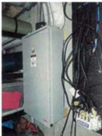
Whole House Generator Transfer Panel Basement
