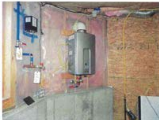
On Demand Hot Water Maker Basement
