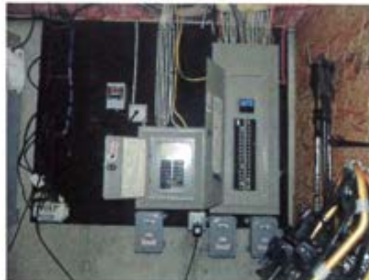
Electrical Panel Basement
