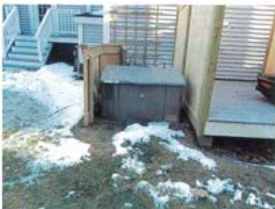
Whole House Generator Rear of Subject
