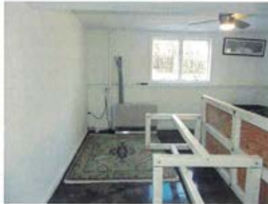
Direct Vent Heater Recreation Room Finished Basement
