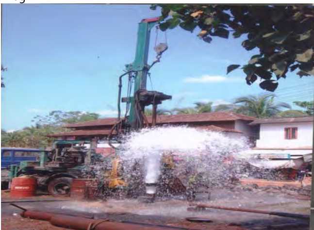
One high yielding PZ constructed at Pangh, Malappuram district with discharge 10 lps, depth 184.50 mtrs and geology: Khondalite.
