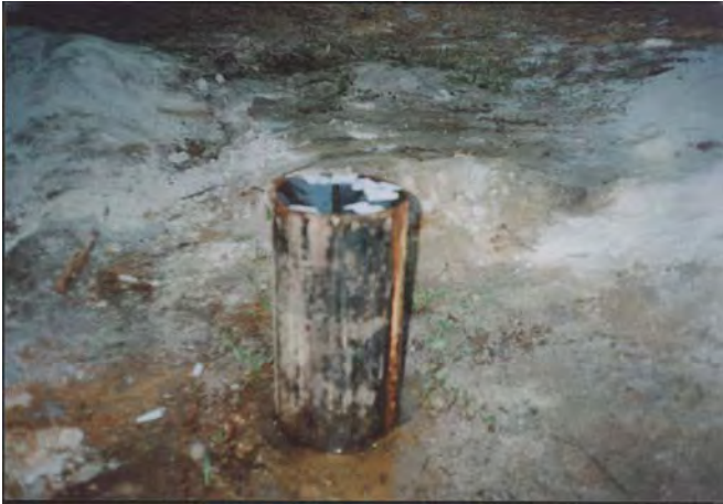
EW drilled at Chithara, Kollam district. The exploratory well is auto flowing (discharge 1 lpm), with a head of 0.95 magl, Depth drilled: 200m bgl and Formation: Leptinite, Khondalite and Dyke.
