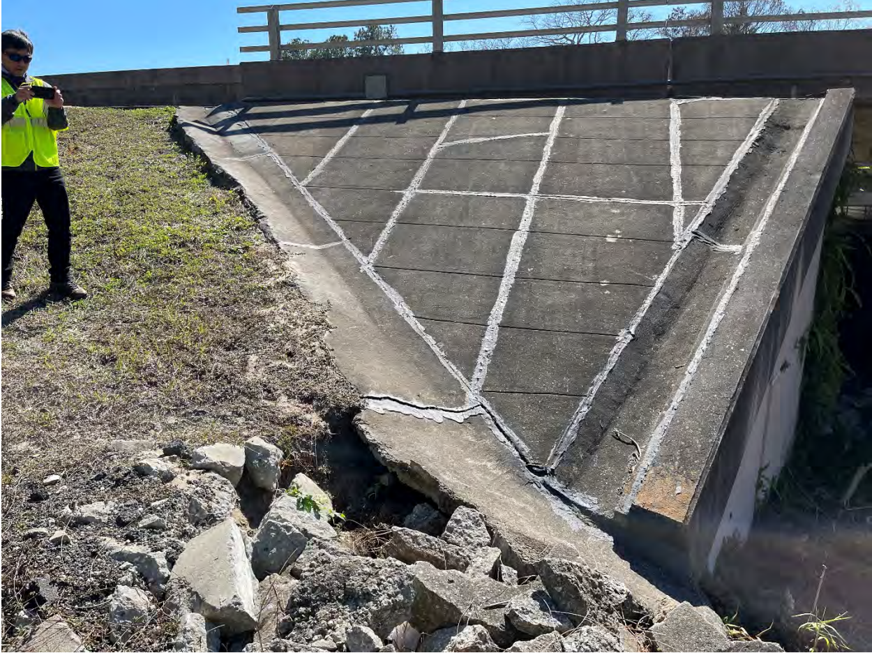
Erosion shown at Little Wekiva Canal Bridge near Lake Lotus Park Entrance
