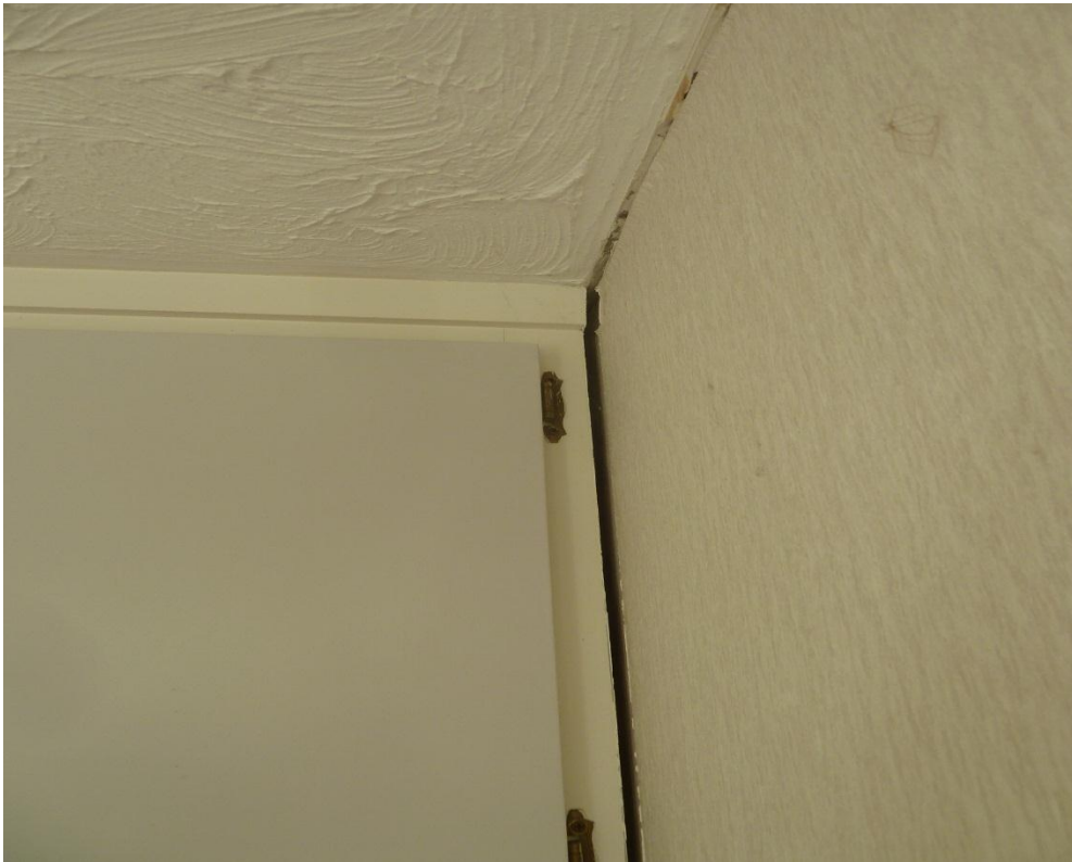
Photo 2: Unit 11 First floor slab pulling away from the tilt slab intermediate wall
