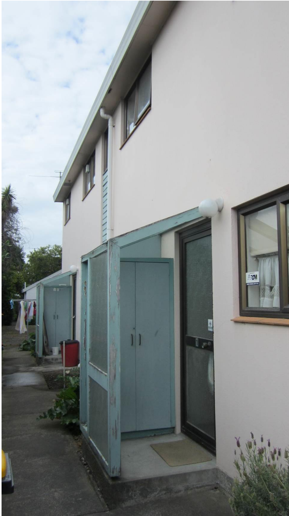
Photo 5: External view of rear of Block A from north-east. Details are typical for Block B also.
