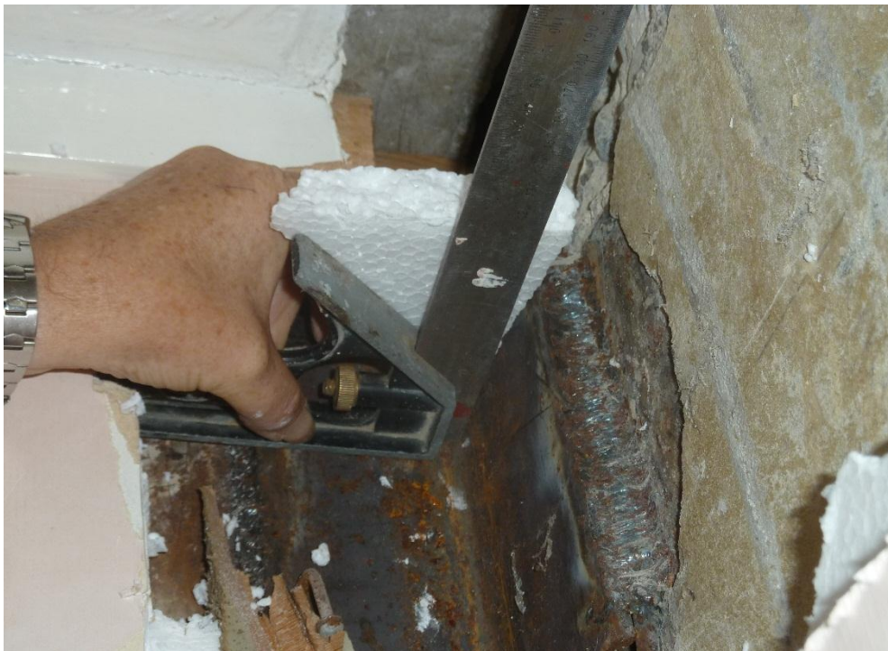
Photo 3: Unit 11 Weld plate no longer 90 degrees
