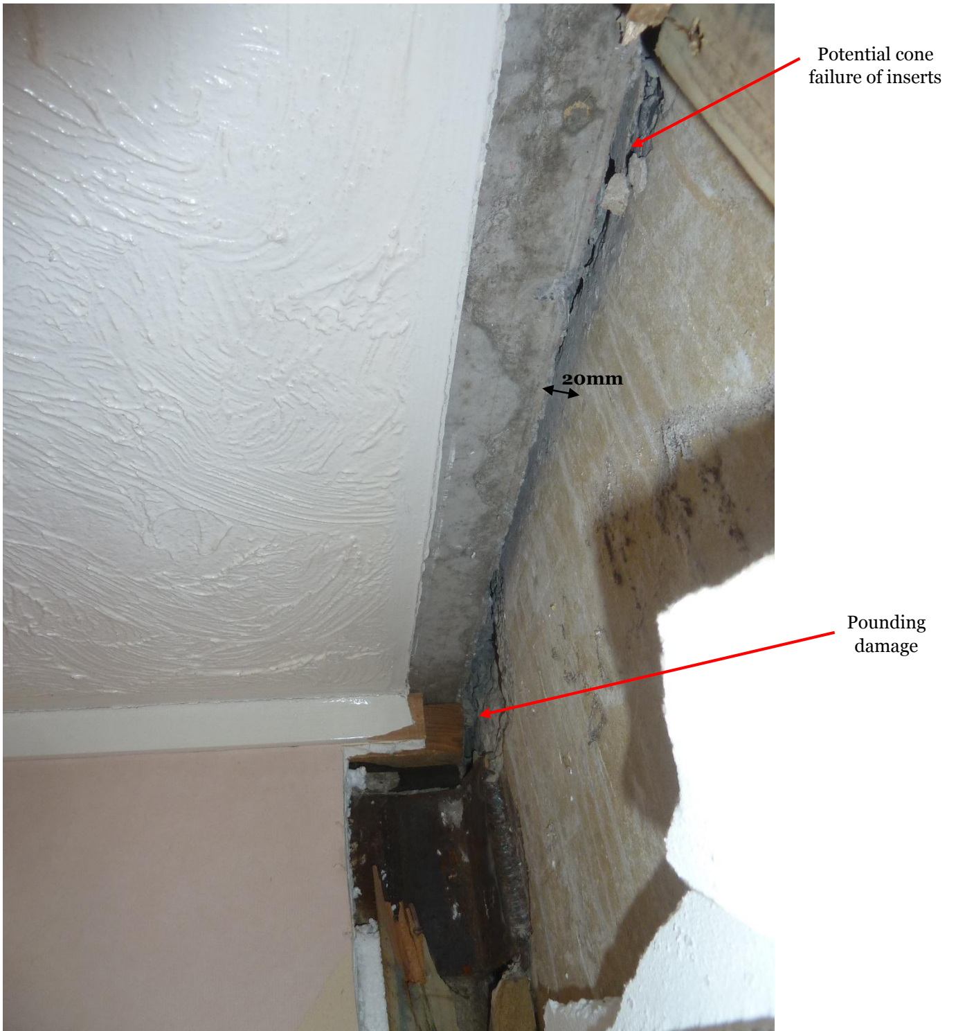
Photo 1: Unit 11 First floor slab pulling away from the tilt slab intermediate wall
