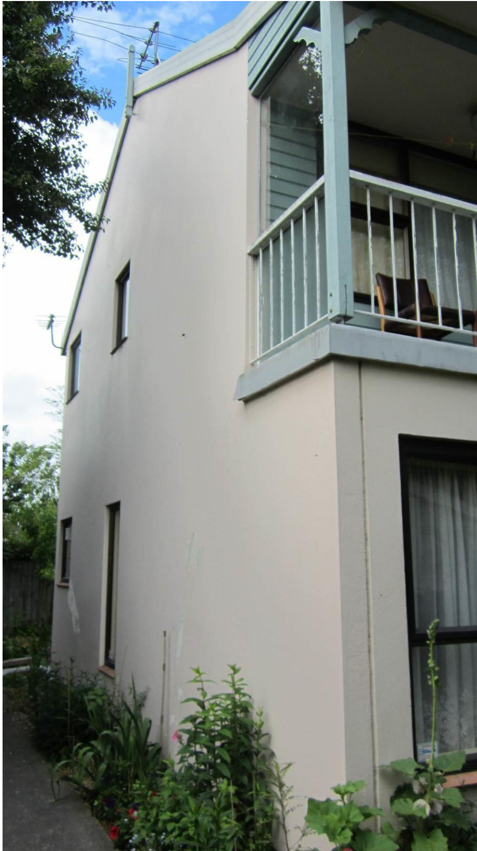
Photo 6: Side elevation of Block B. Detail is typical for both ends of Block A and Block B. (0.1mm crack width)
