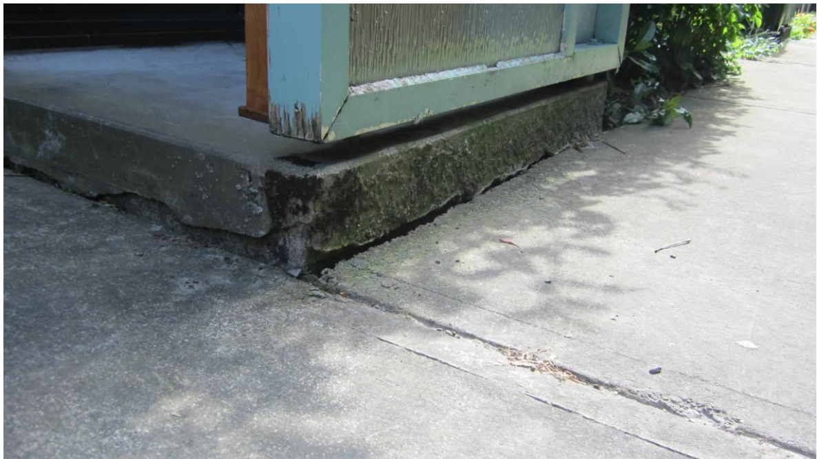
Photo 16: Rear porch entrance and pavement (typical for Block A, Block B and Block C).
