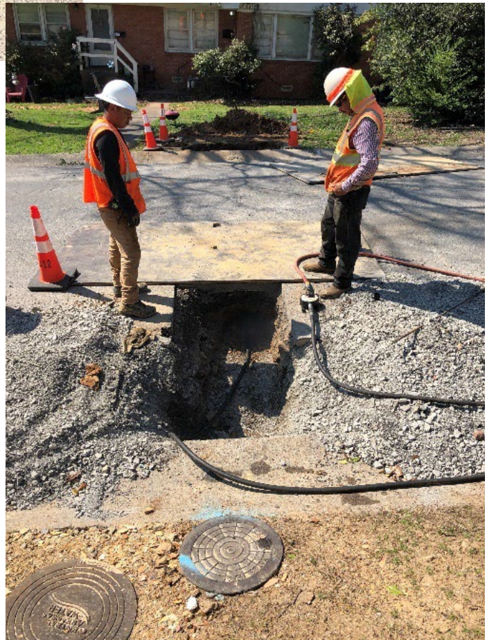
Service line being placed under the street to serve a meter on the "long" side of the street from the new water main. A pneumatic boring tool is being used to punch a line under the pavement without cutting all the way across the street.
