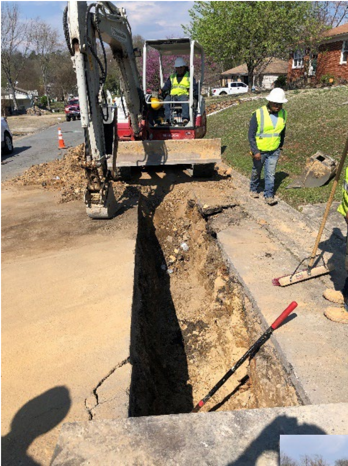
Open-cut trenching along Blackwood Road. The new pipe is being installed just inside the outer edge of the asphalt street surface. It is difficult to see in the photograph, but the trenching is hard and slow due to rock.
