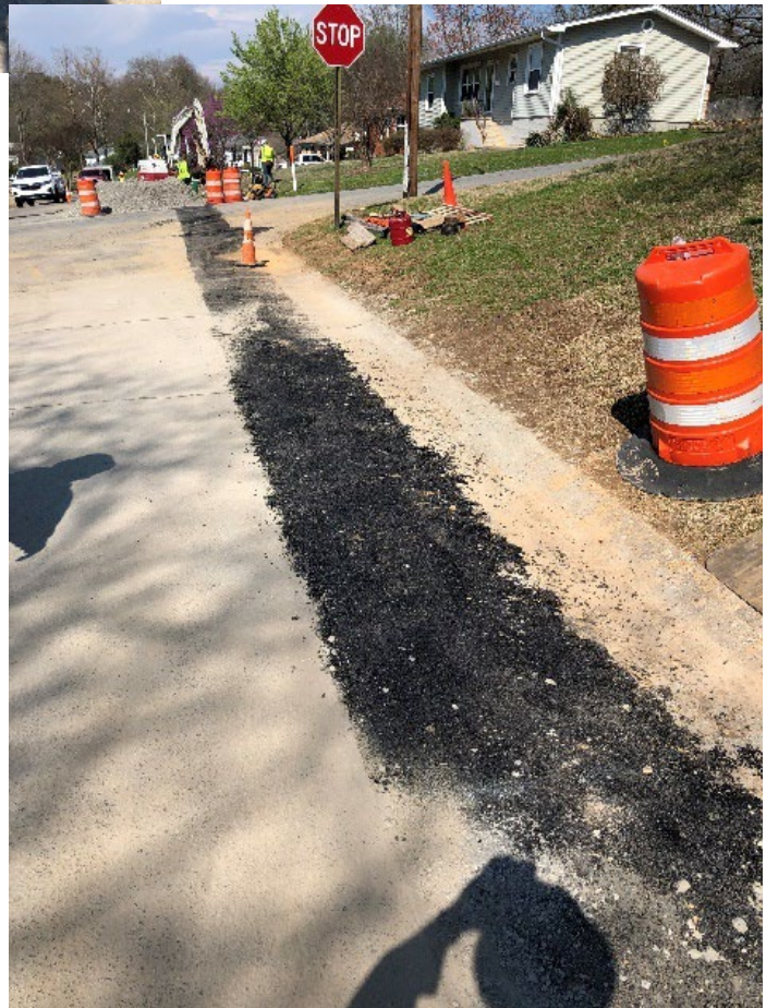
After the new pipe is laid, a temporary street repair is completed. The repair consists of removal of the native material, backfilling the trench with 100% crushed stone (compacted), and topping the trench with cold-mix asphalt. The permanent repair will be made at a later date.
