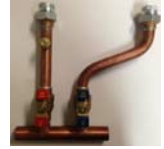
Boiler Piping 1-1/4" header for HC & DC boiler
