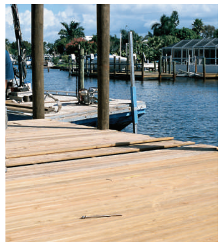
Elevated Service / Severe
