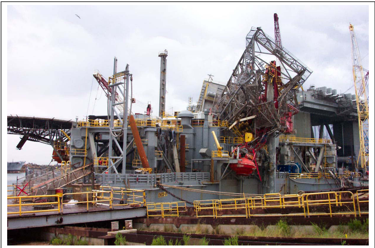
Figure 33: Photo showing the derrick collapsed.
