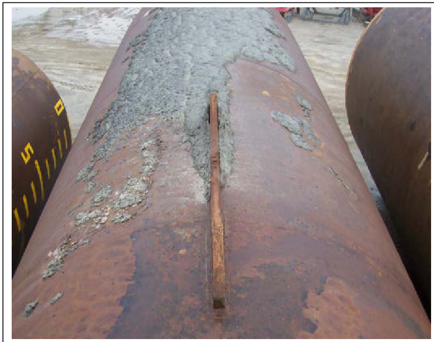
Figure 18: Shows the Damaged Padeye on the Suction Piles. The padeye angle was about 45° at the time of failure.
