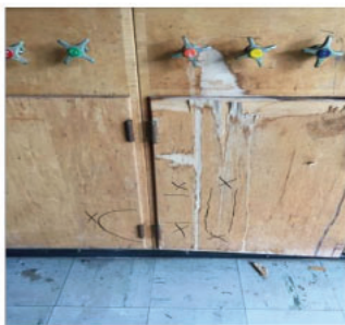
Figure 1: Building 830 lab 3. Temporary black markings for contamination on hinge
