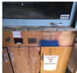
Figure 2: Building 830 lab 3. Temporary black markings for contamination just below hood and permanent marking of previously known contamination
