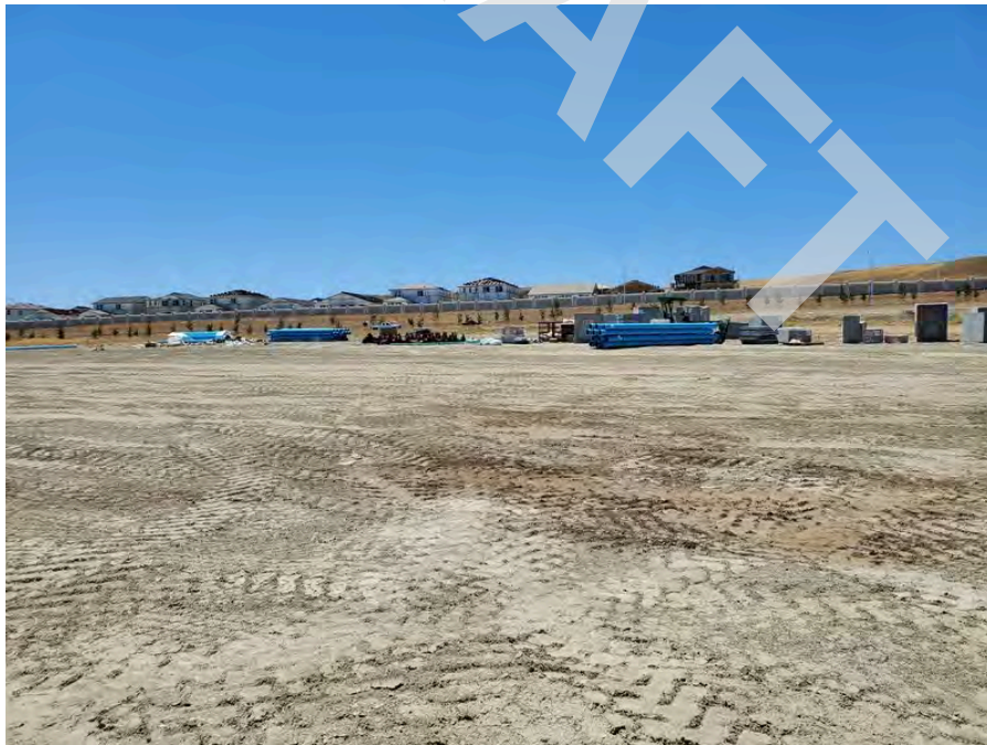
14 - Another view of construction materials located in the center of the Site.
