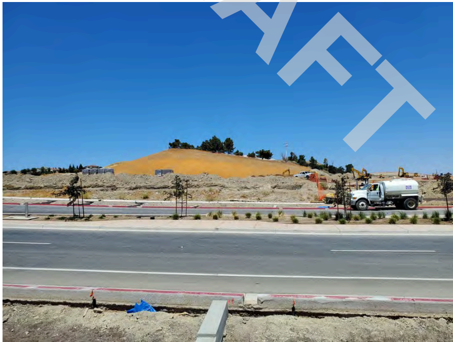
6 - Vacant land under development beyond Laurel Road to the northwest of the Site.
