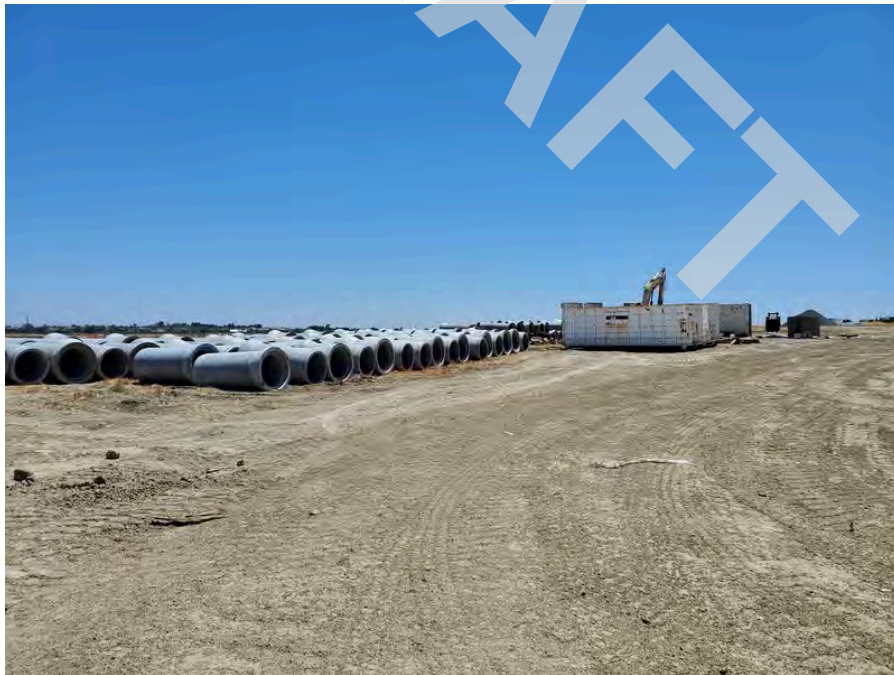
8 - Additional construction materials on the northeastern portion of the Site adjacent to the Route 4 on ramp.
