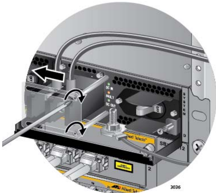
Figure 112. Closing the Plastic Cover over the Terminal Connectors
