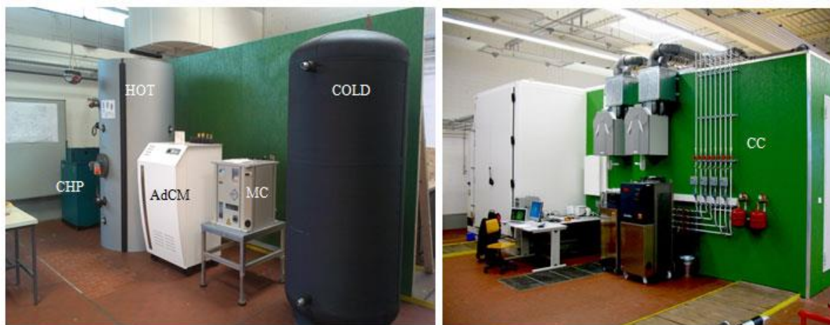
Figure 3: Trigeneration unit and climate chamber (CC) at the Institute of Energy System Technologies (INES)
