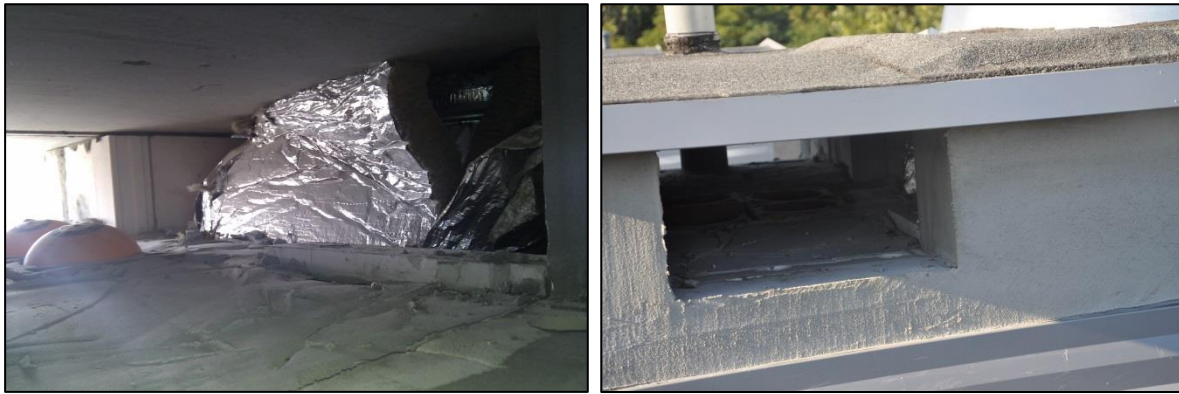
Figure 8: Chimneys top with gaps between chimney walls and ventilation duct
