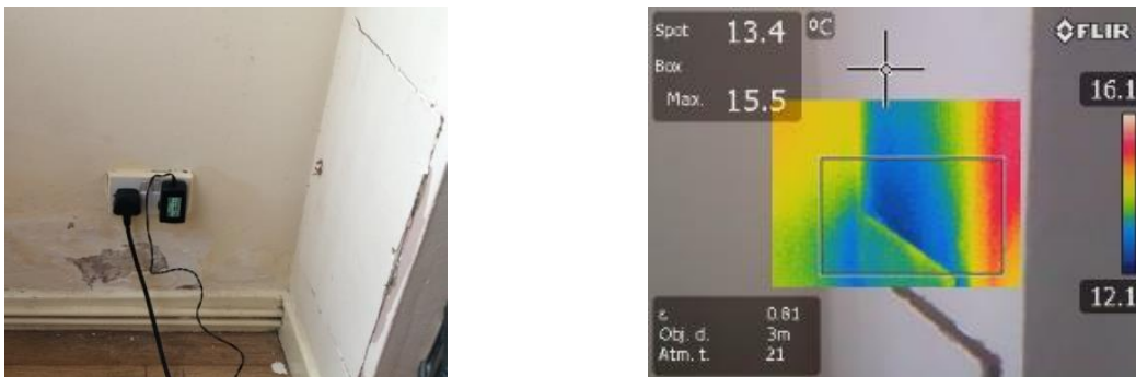
Figure 6: Photograph and thermographic image of a loosely installed plasterboard panel in house No. 2.
