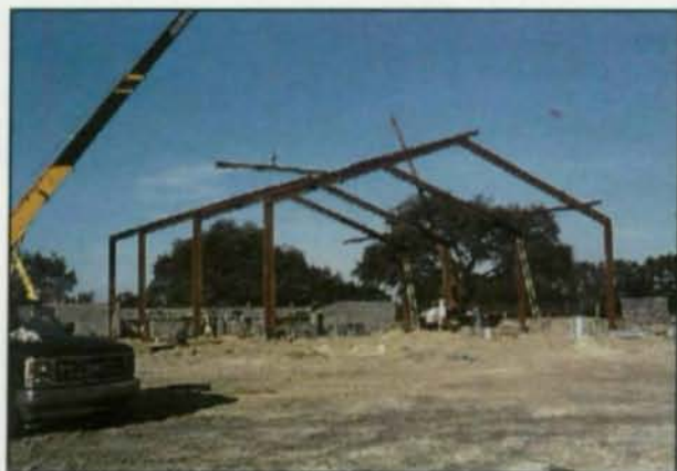
A gable frame fabricated from W16 sections provided an 80-ft. clear span for a gym at the Newberry Middle School at a lower cost than a similarly sized metal building.
