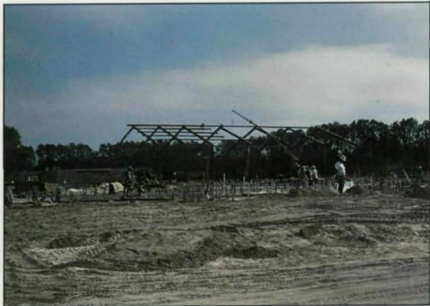
Pictured is one of the three buildings at the Prairie View Elementary School, which were fabricated from W12 sections.
