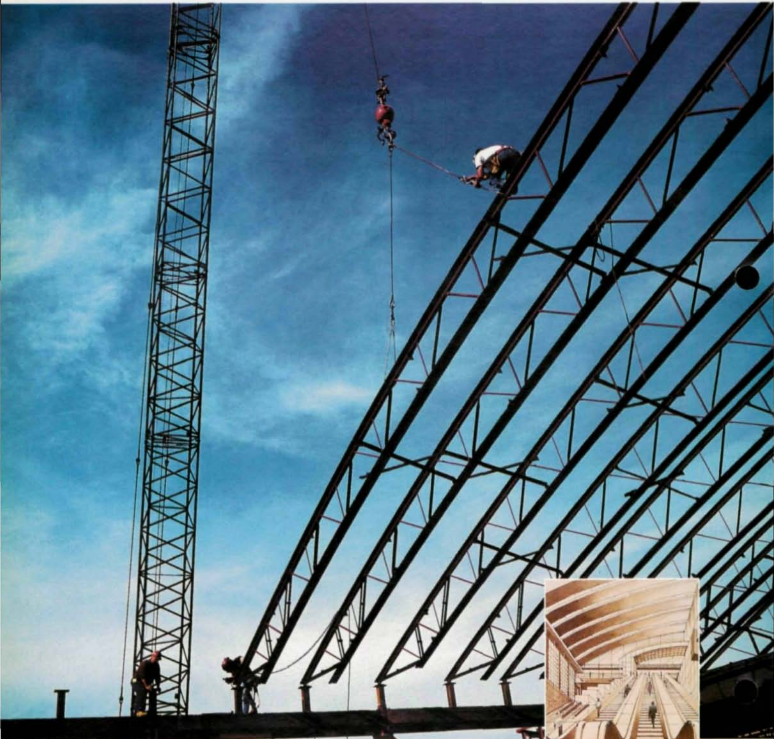
Arched chord joists top the Arrivals Hall, International Concourse, Hartsfield Atlanta International Airport
