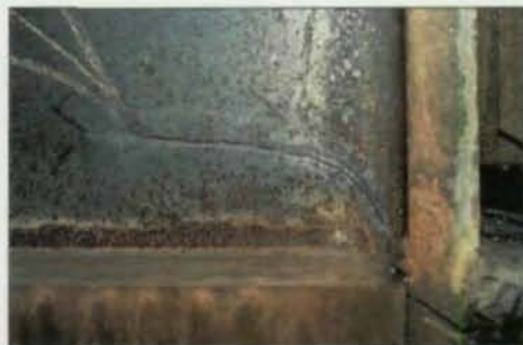
Some steel structures exhibited localized weld failures and flange cracking. The welds have already been repaired in this example.
