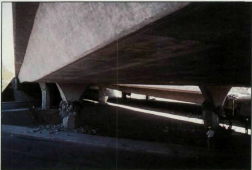
Damage to concrete overpasses in 1971 (top) was similar to the damage suffered in 1994 (above). Photos courtesy of EQE Engineering.
