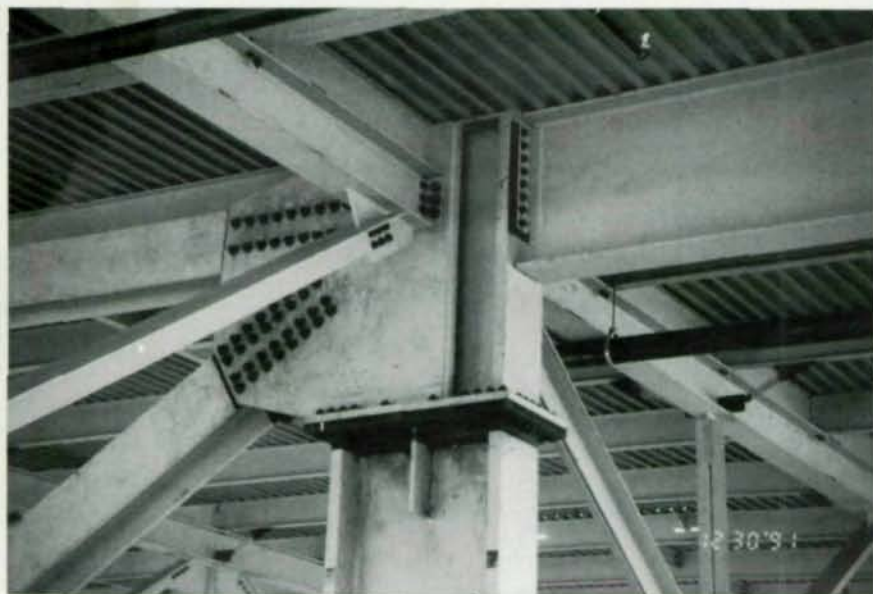
The magnitude of the loads resulted in chord forces as large as 1,635 kips. After analysis, W14 shapes with a yield strength of 50 ksi were selected as optimum for the high axial loads in the truss chords. For the top chord, a 1 7/8" cap plate was welded to the column and a specially fabricated piece of the W14 column sits on the cap plate.
