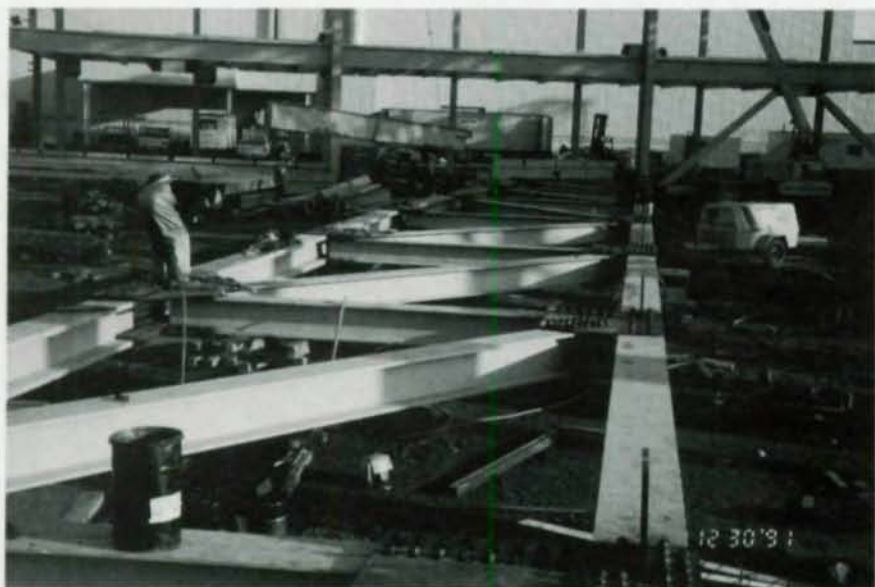
A nominal truss depth of 16' was identified as the most economic design based on simple-span gravity load analysis. Axial column loads due to dead and live loads are as large as 600 kips, while the gravity loads can reach 1,635 kips.
