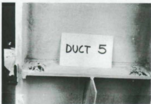
Fig. 24. Continuity Plate Between Column Flanges. Shear Plate for Connecting Beam at Right Angles to the Test Specimen is in the Middle of the Panel Zone.
